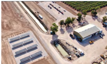
Huddersfield solar installation
